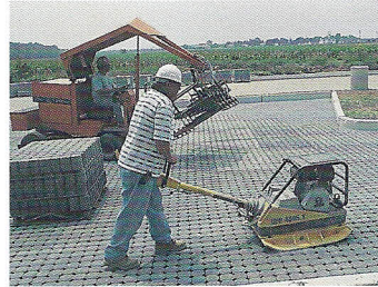
Aggregate base and subbase are spread and compacted; pavers are delivered ready to install. After placement, joints and/or openings are filled with small aggregate and pavers compacted at this Walmart in Rehobeth Beach, DE.
